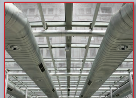
Find blockages or broken registers in A/C ductwork
